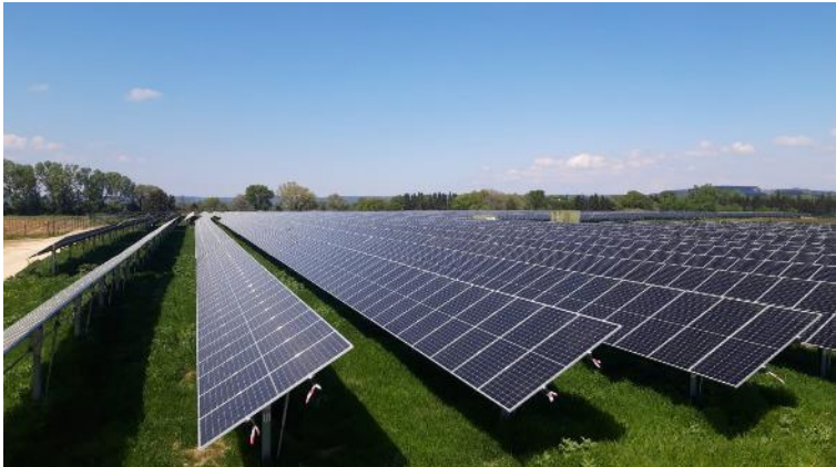
Sernhac – 5 MWp – France
