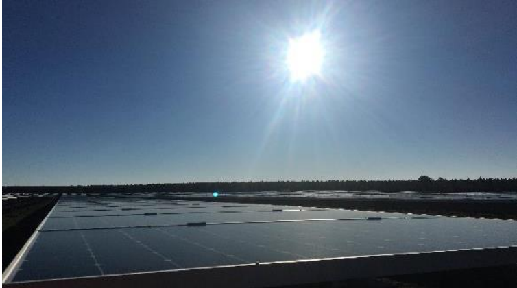
Reaup-Lisse – 15 MWp – France
