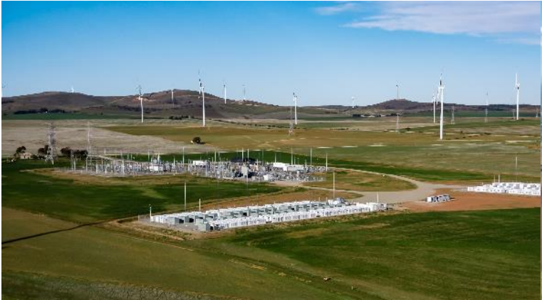
Hornsdale Power Reserve - 150 MW – Australia
