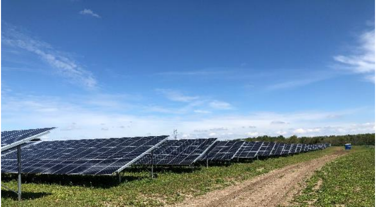
Mer - 15 MWp - France
