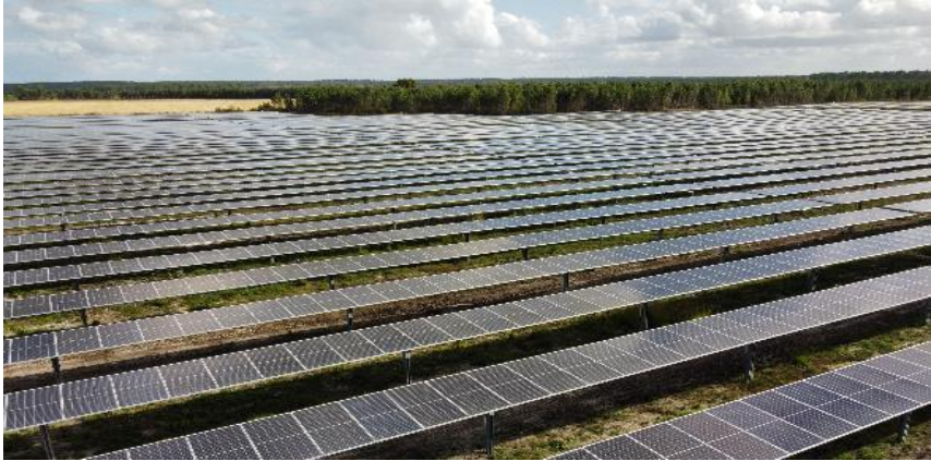
Arue 3 – 16 MWp – France
